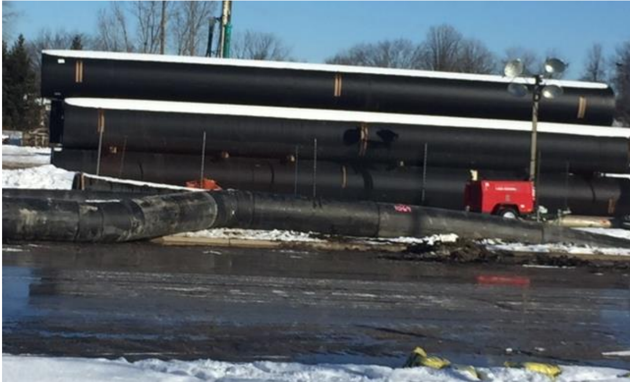
48-inch diameter bypass pipe
