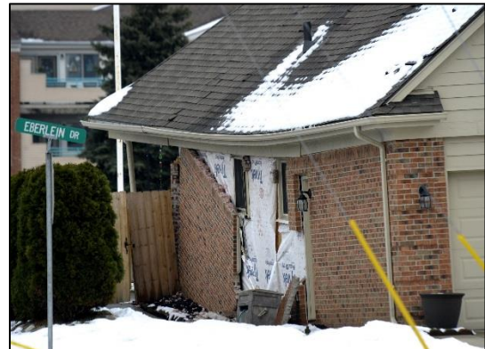
Home damaged by collapse of sewer line.
